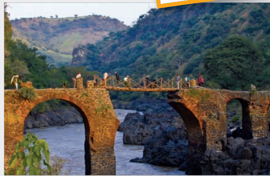
Previous spread: villagers rebuilding the Sebara Dildiy bridge. Clockwise, from top: A new steel truss is tested in 2002; a National Geographic article about Frantz; a makeshift wooden bridge in 2007; crossing the Nile by rope, after floods destroyed the 2002 steel bridge.
