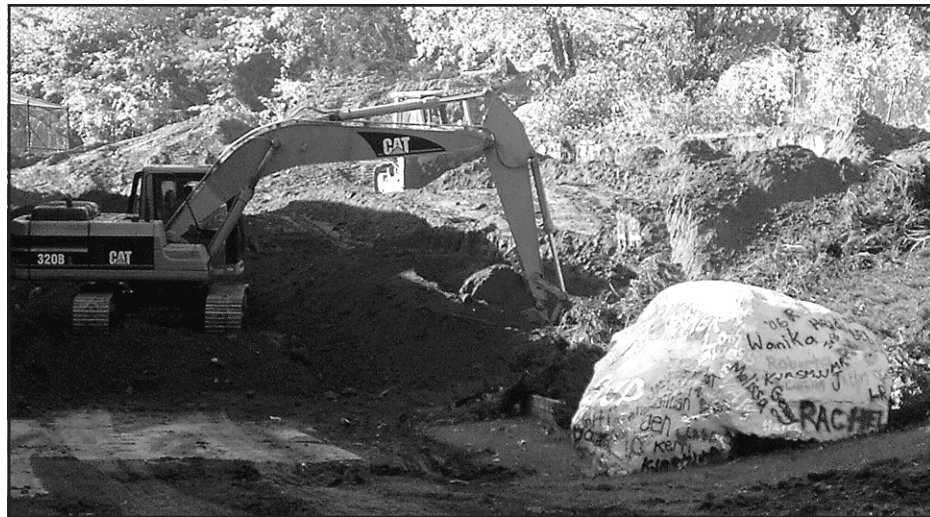
The construction and digging behind the Blind Brook school building has already commenced. Photos by Emily Brackman
