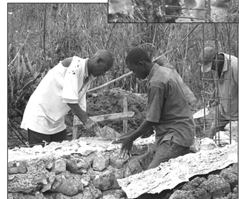
Men help with the construction of the new school at St. Paul's Episcopal Church.
