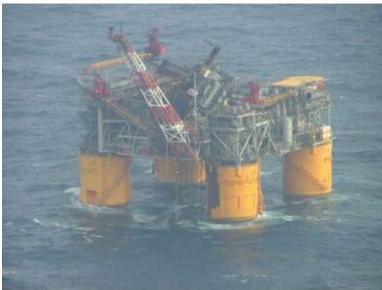
Mars TLP after Hurricane Katrina
