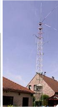
A steel amateur radio antenna mast
