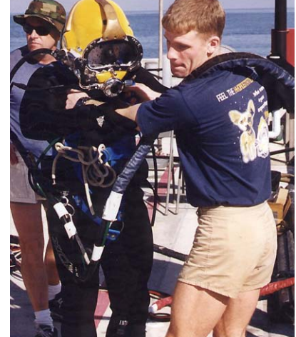
Detachment ONE in San Diego preparing to launch divers during pier repair operations. Photo by Combat Camera, Atlantic.
