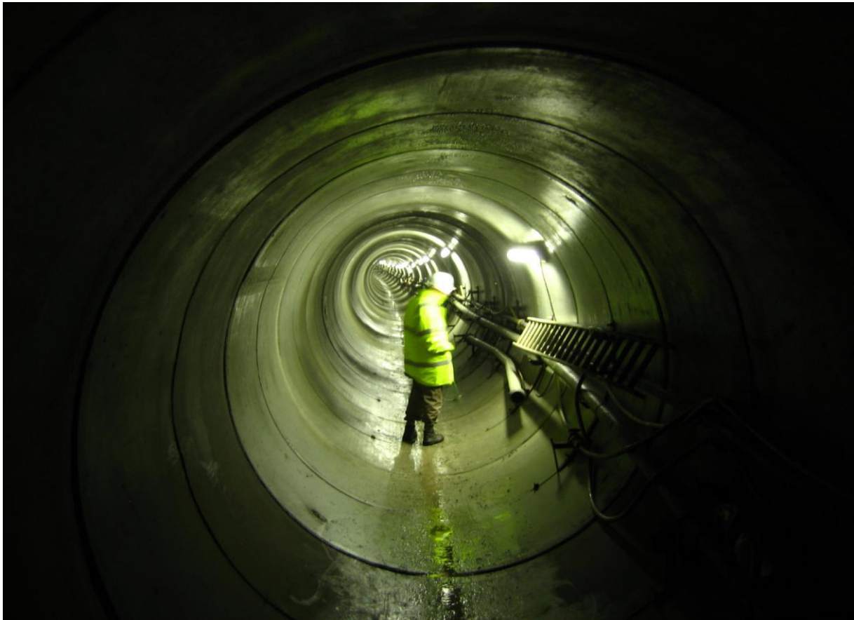
Inside the Liffey Services Tunnel
