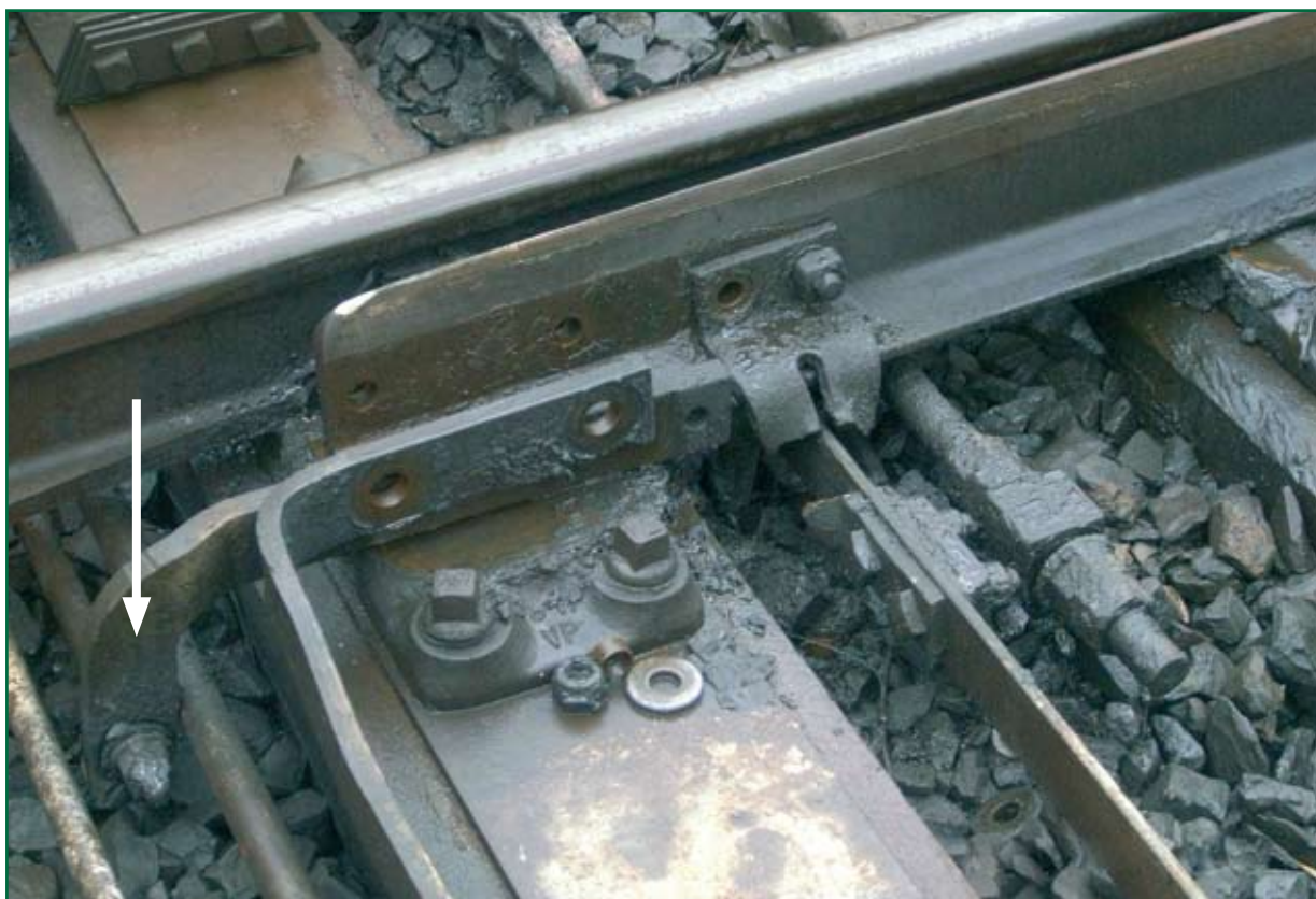
Figure 15: Left-hand switch rail toe showing switch rail extension piece (arrowed)
