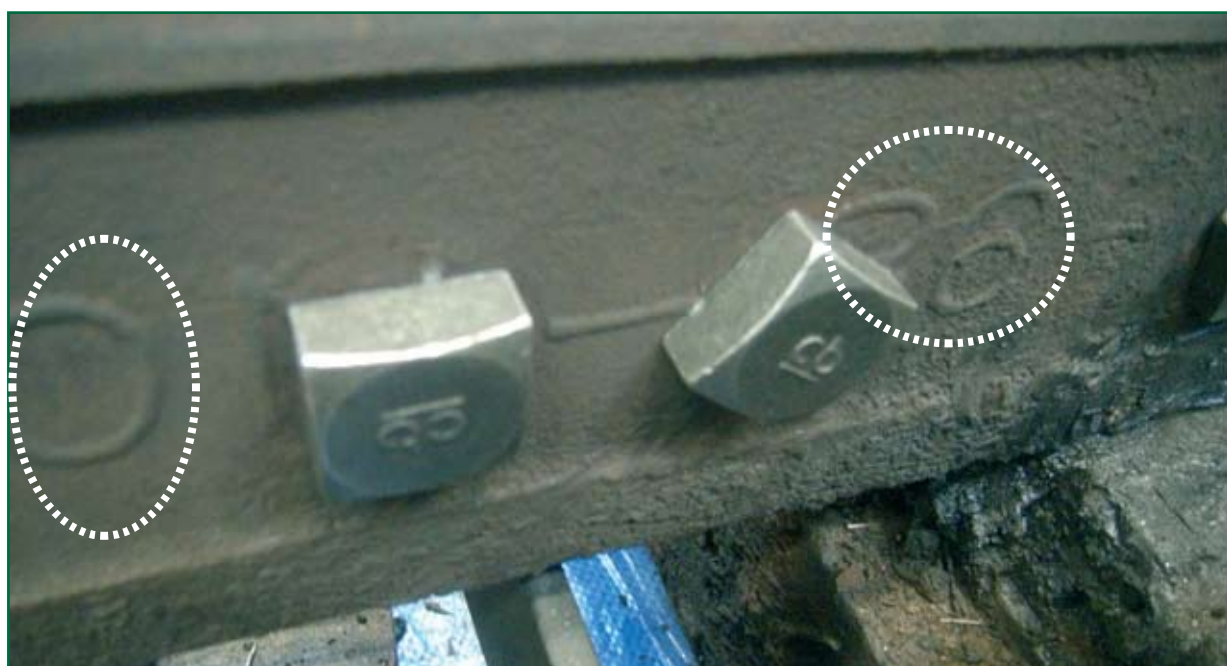
Figure 11: Rail branding on left-hand switch rail (Note: new bolts added for testing purposes)
