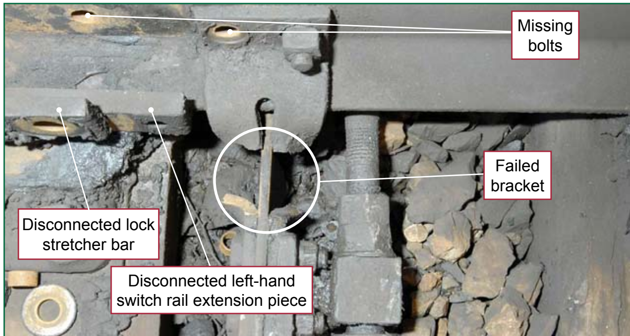
Figure 16: Failed bracket first permanent way stretcher bar
