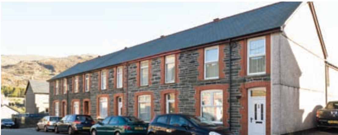
Loss of chimneys has damaged the original rhythm of the terrace (Crown Copyright: RCAHMW).
