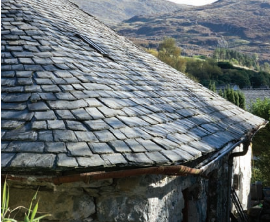
Left: A fine example of slate roofing at Yr Unicorn (Crown Copyright: RCAHMW).
