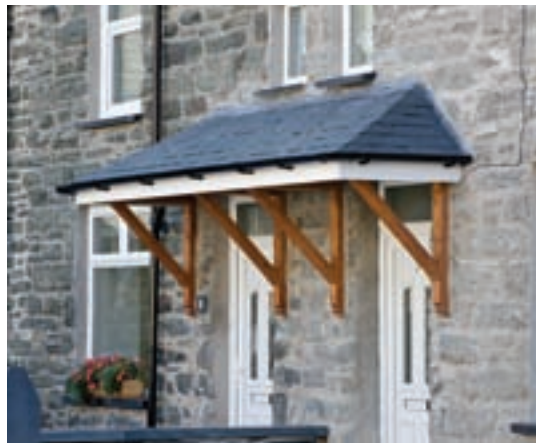
Park Square: Picturesque detail has been lost in the modern replacement of porches (left) and gable detail (below) (Crown Copyright: RCAHMW).
