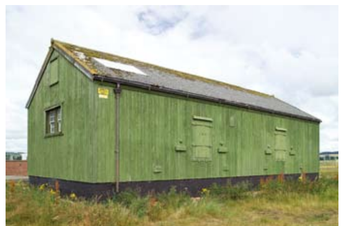
Naval gunnery training room known as the 'Gunnery Gym', showing gunports in south-east side, Barry Buddon. DP004830
