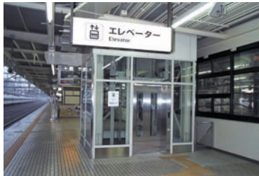
Wheel Chair-Accessible Elevators
