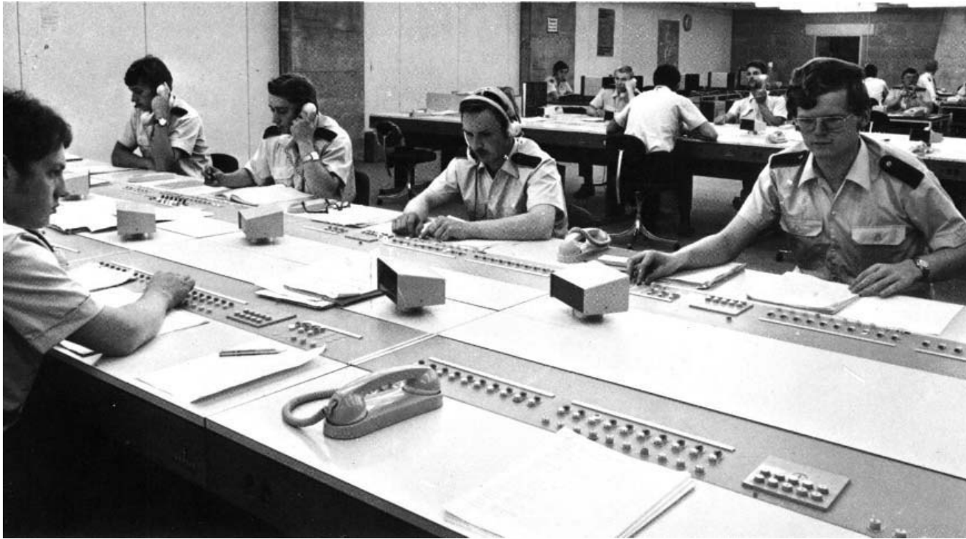
The large telephone exchange in Olympic Stadium (20 operators for ca. 2,000 extensions, 390 trunk lines, 186 cross connections to the sub-exchanges)
