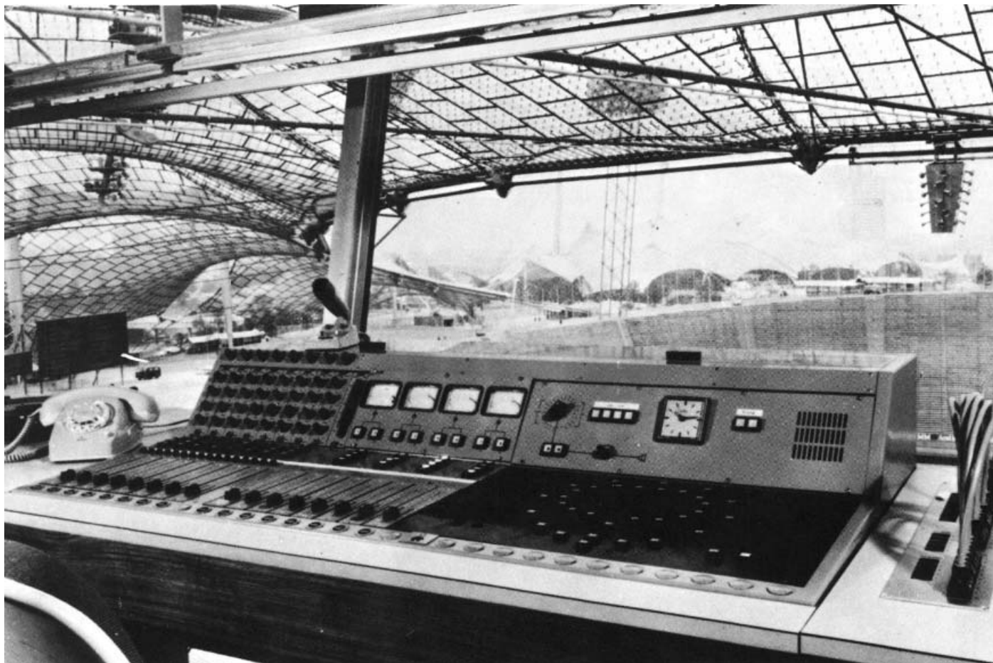
Public address equipment in Olympic Stadium control room
