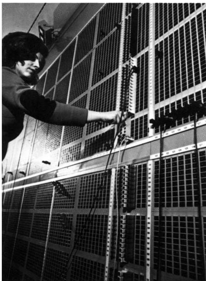
Cross grid dividers in the control center
