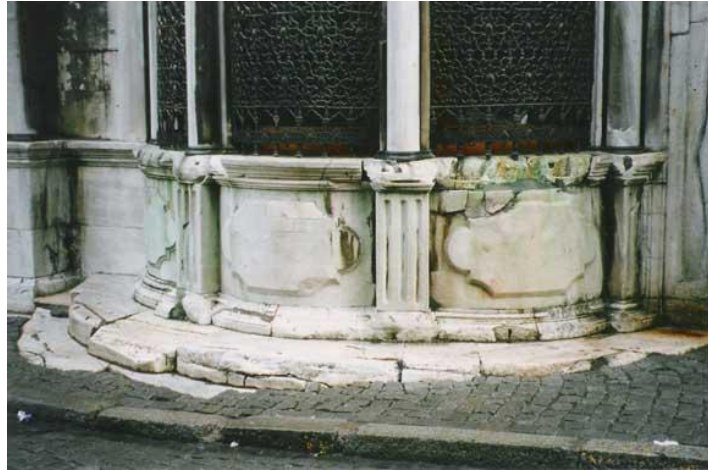
Figure 6. The situation of the balustrade elements before the restoration (Saglar Onay archive)
