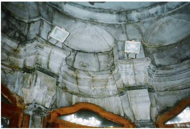
Figure 11. The Interior of The Sebil of Nuruosmaniye - The situation before restoration (Saglar Onay archive)
