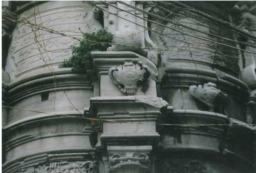
Figure 13. The Inscriptive cartouches of the Sebil of Nuruosmaniye – The situation before the Restoration
