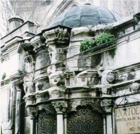
Figure 5. The situation of the upper structural elements before the restoration (Saglar Onay archive)
