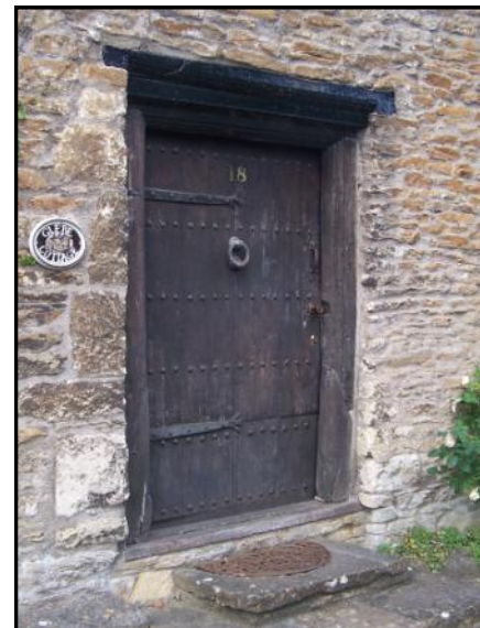
Planked door with rivet heads and strapped hinges at no.18 Church Hill
