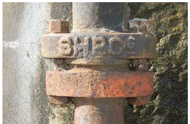
Figure 21. HP Joint on Remnant 4” Main, Sydney.
