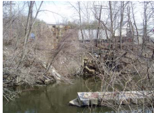
Figure III.6: Remnants of B&W Bridge over Blackstone River
