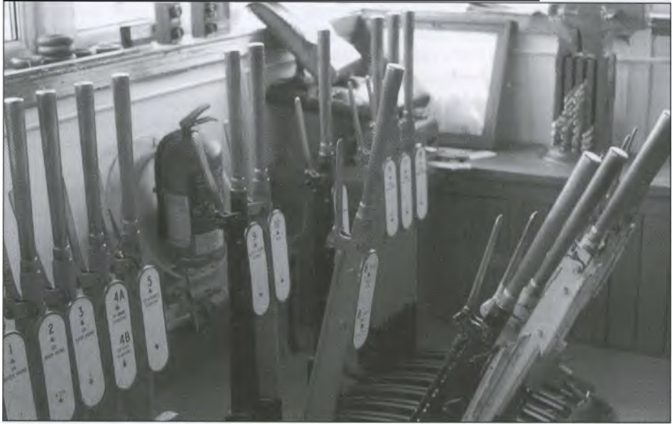
Manual signal cabins, like this one at Enniscorthy, are now an endangered species. In the background is a block token instrument and a keen eye will note that two of the levers, by having a halfway position, can operate two signals each. [I Pryce]
