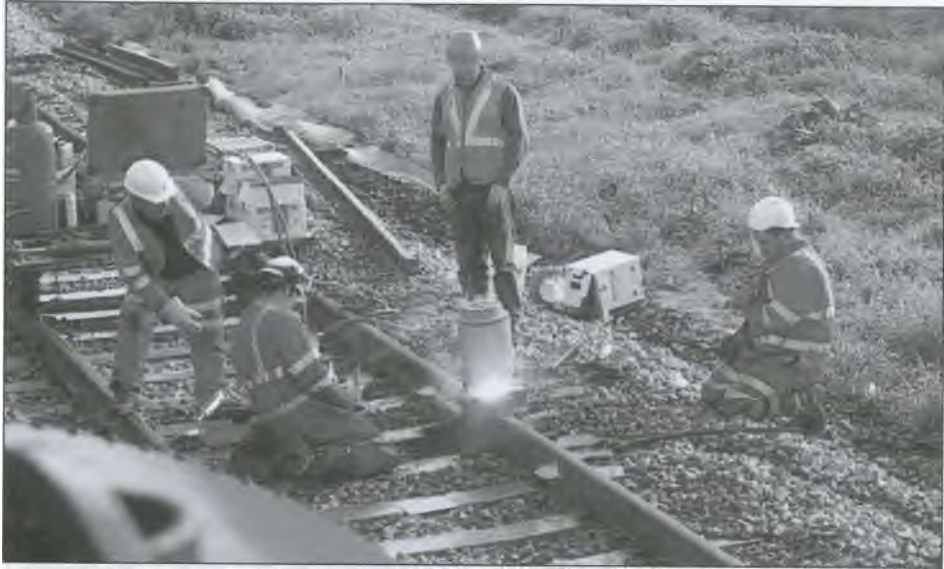
The Thermit welding team in action. Since they are at Greenisland it will be some weeks before shellfish become available. [I Pryce]
