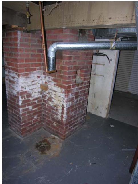
Figure 22 – 131 Trafalgar Rd., detail view of basement interior of showing centre brick chimney foundation
