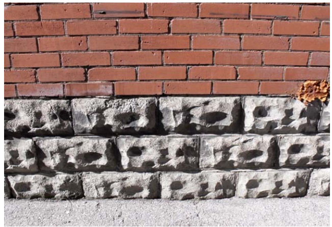
Figure 17 – 131 Trafalgar Rd., detail view of exterior masonry showing smooth bricks & rusticated cement block foundation
