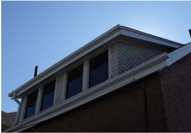
Figure 16 – 131 Trafalgar Rd., detail view of rear (east) dormer showing original wood shingles
