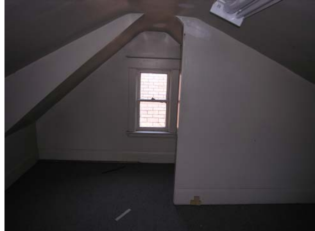
Figure 20 – 131 Trafalgar Rd., detail view of interior of third floor showing baseboard & window casing
