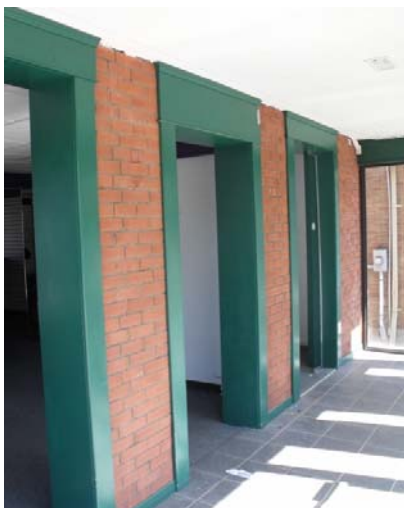
Figure 18 – 131 Trafalgar Rd., detail view of west (front) façade inside enclosed porch showing alterations with openings
