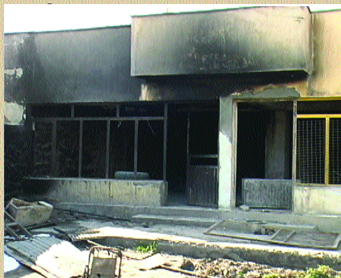
Damaged seed laboratory in Badam Bagh.
