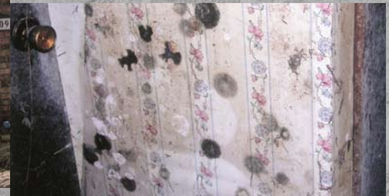
Debris and moldy walls greeted Scivicque in her return trip home. She had to break a window to get in.
