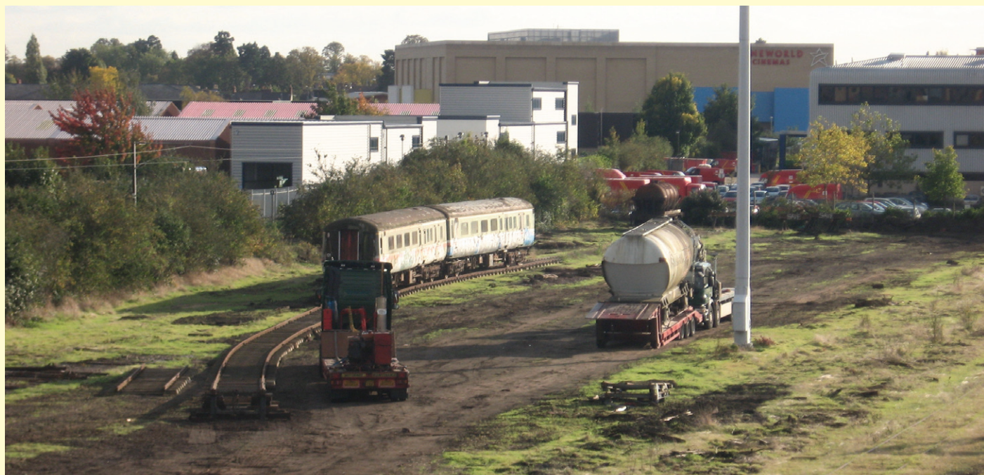
▲ As part of the redevelopment of Cambridge station, the sidings opposite Platforms 1 and 4 were removed at the end of August. This week it was the turn of the stabled stock (a three-axle tank, two cement tanks and two BR MK2 coaches). A familiar sight at Cambridge for many years, the stock remained on a short stretch of track until this week. Temporary track was installed to move the stock onto lorries for road transport. This photo was taken from the Cambridge pedestrian footbridge and shows the two coaches and three-axle tank waiting to be moved, the remaining cement tank waiting taken by road. Thomas Blampied
