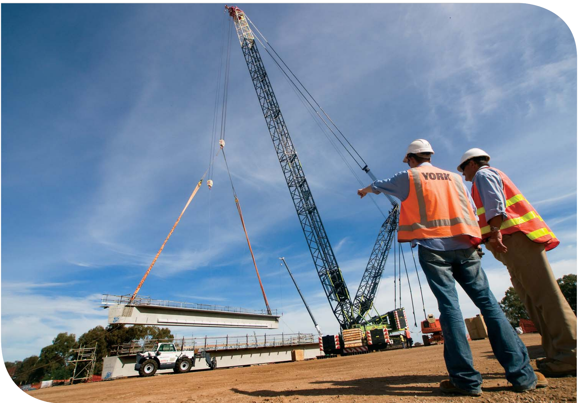
> One of Australia's heaviest lift cranes helps to complete the last two bridges on the Northern Expressway.
