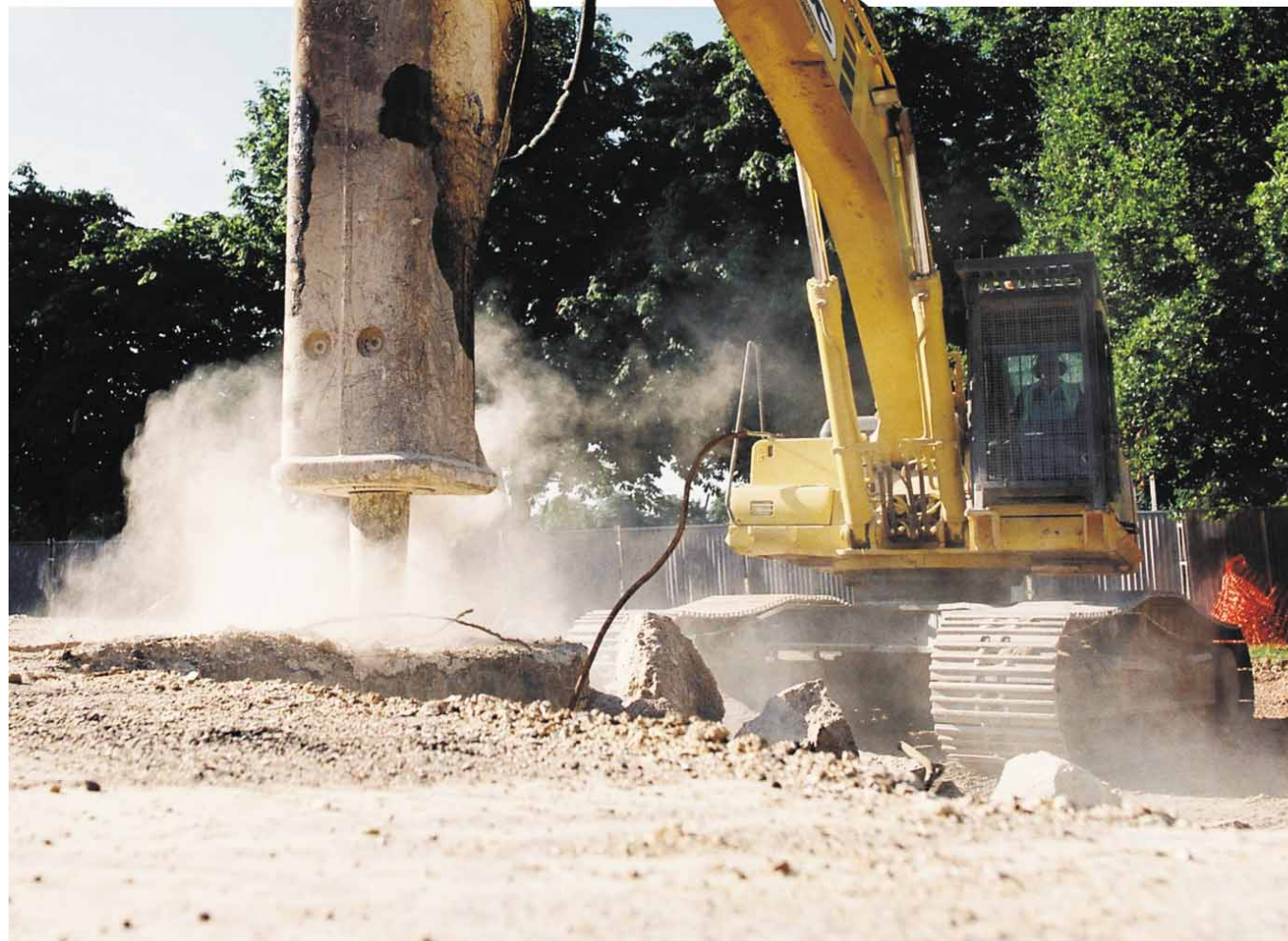
Right: Land restoration at the eastern end of the site will pave the way for delicensing.
