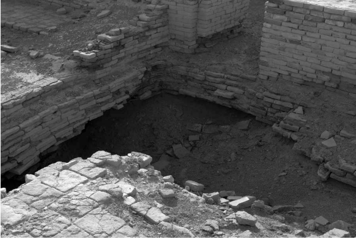
Fig. 20. Collapsing brickwork in the area of the Third Dynasty of Ur tombs
