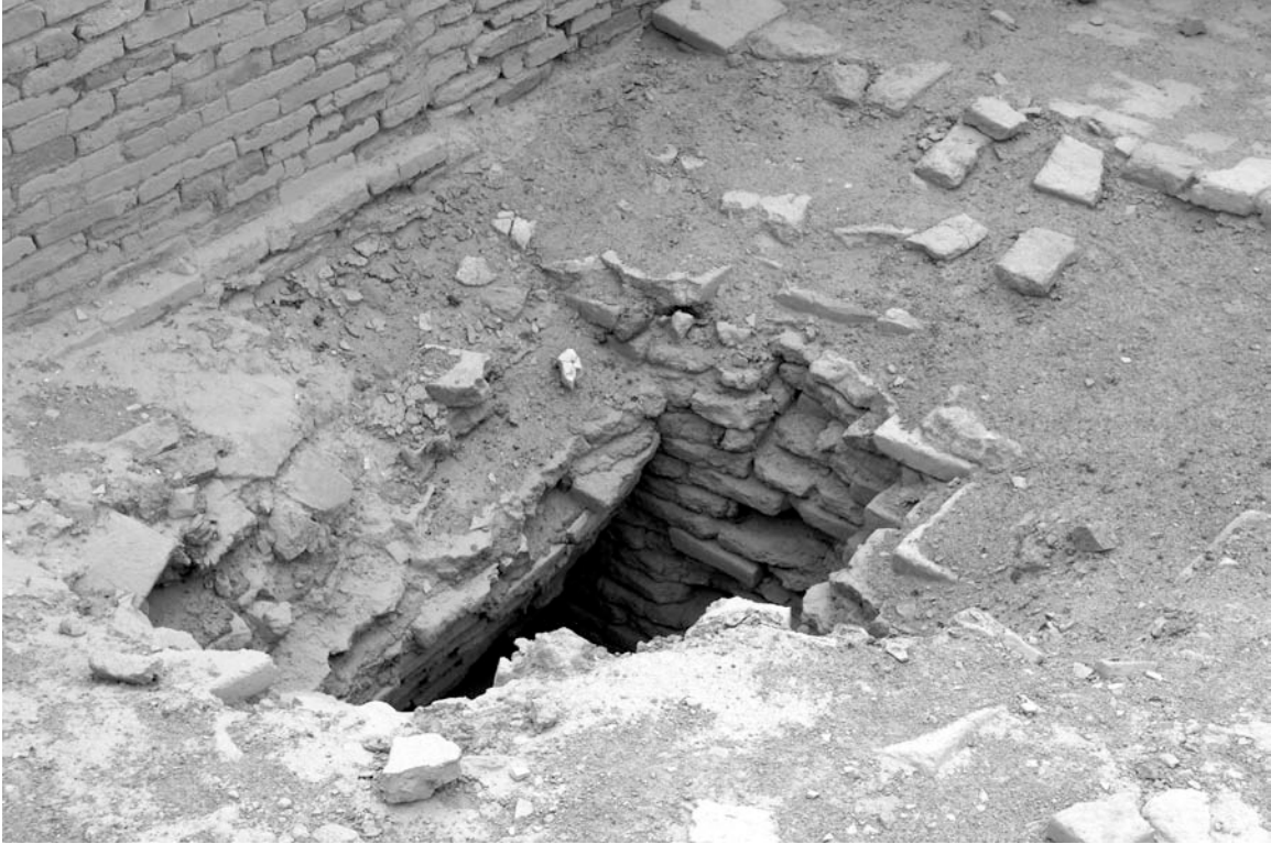
Fig. 22. A collapsed section of the roof of a Third Dynasty of Ur tomb
