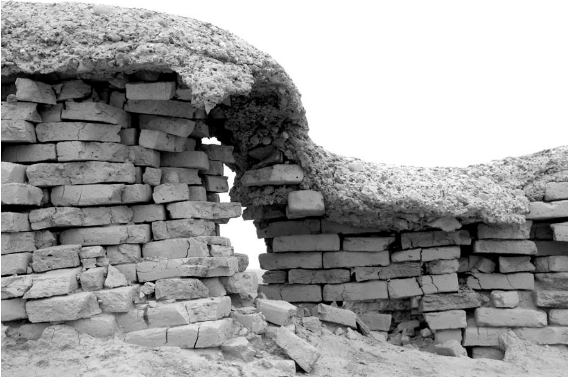
Fig. 18. A protective layer of concrete placed over the top of the walls of the E-Dublal-mah temple
