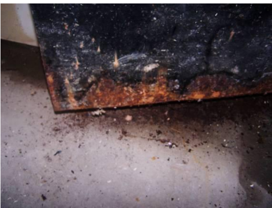
(Fig 17-The erosion on the vault door)
