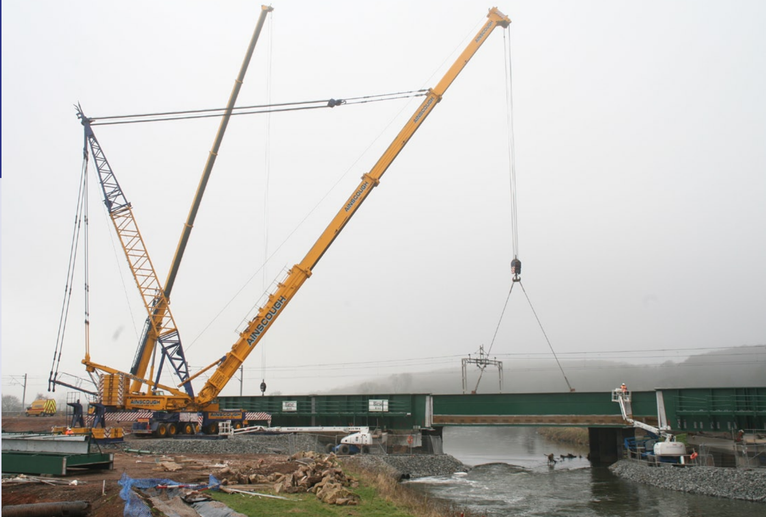
ABOVE: Another part of the Trent Valley Four Tracking project was lifted into place, literally, on 18th February, when one of the new bridges, which will provide two additional tracks between Tamworth and Armitage with Hansacre, was lowered into place over the River Tame. The existing two track railway will be diverted on to the new bridge, after which the existing bridge will be replaced by a second new bridge, which will carry the additional two lines. A 1000 tonne capacity crane lifted the girders, which make up the structure into place. The bridge will consist of three spans making up a bridge of length 92 metres and 12 metres wide. WILF SMITH
