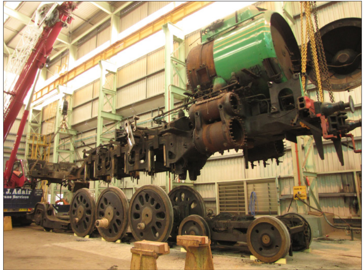
▲ A mobile crane carefully lifts the frames and smoke box of Australian Pacific No. 3801 off the wheels at the New South Wales Transport Museum in Thirlmere. NSWTM
