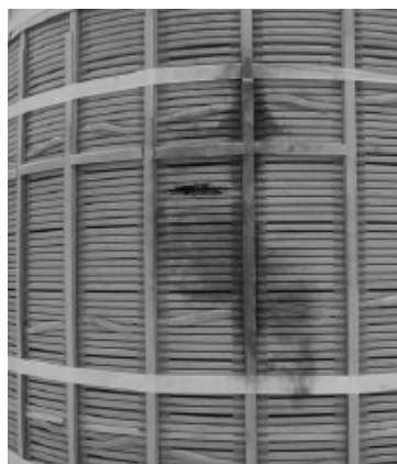
Fig 9: Damaged HV winding of Ruacana GSU transformer
