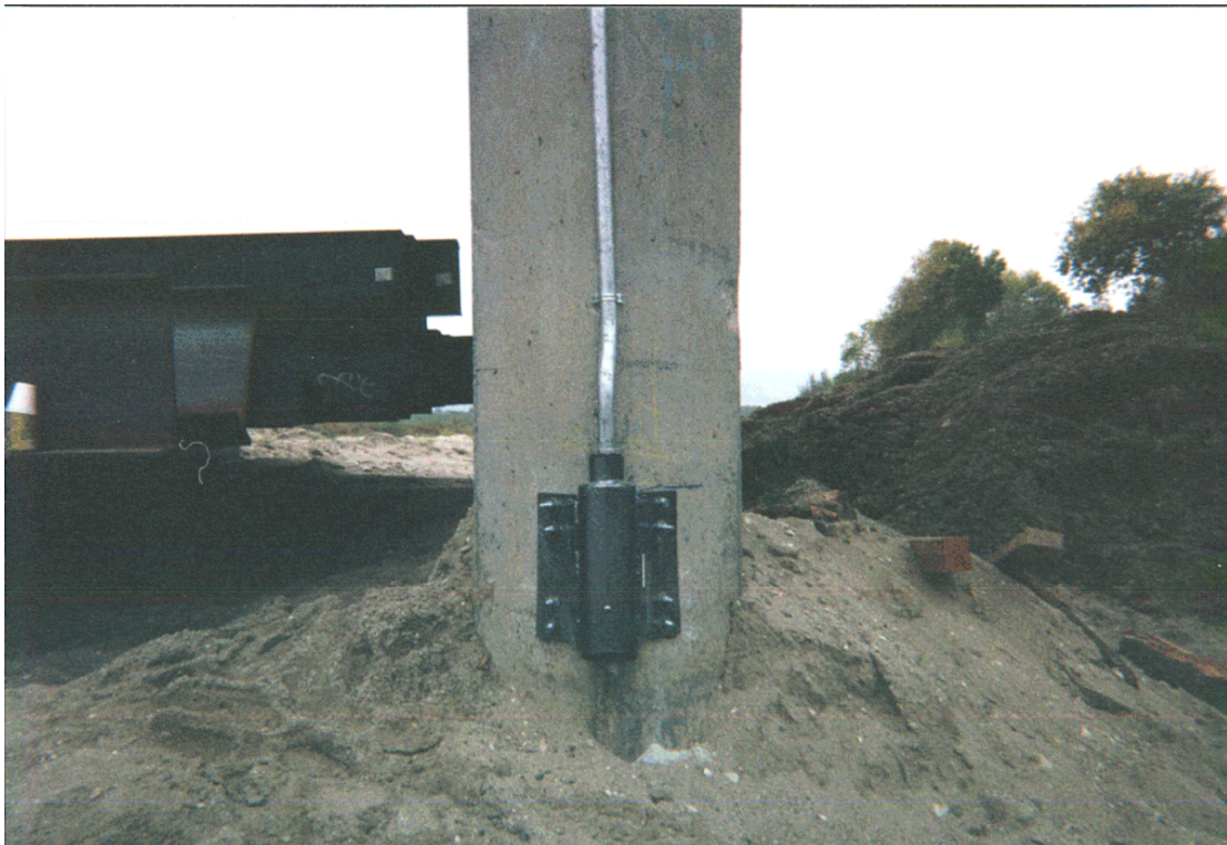
Figure 7.14. Close up of sonar scour monitor on Salinas River bridge near Soledad, CA.
