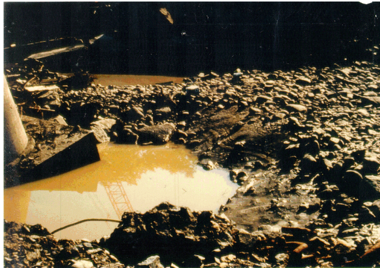
Figure 8.2. Pier scour holes at Schoharie Creek bridge in 1987. Pier 2 in the foreground with pier 3 in the background. (2)
