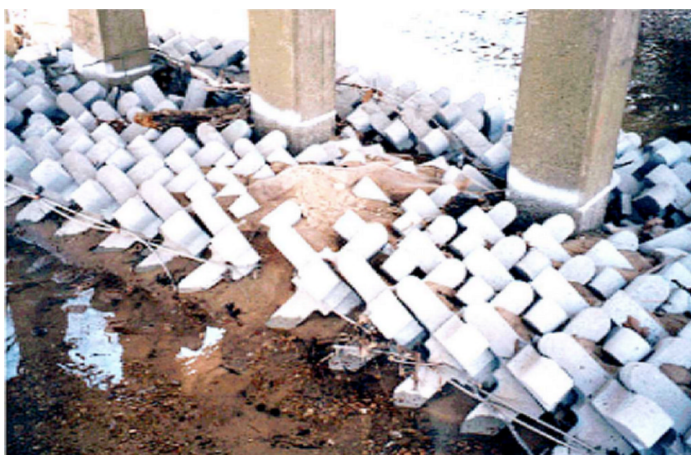
Figure 6.13c. Close-up of armor units after several flow events at Bridge 133, Graves County, KY
