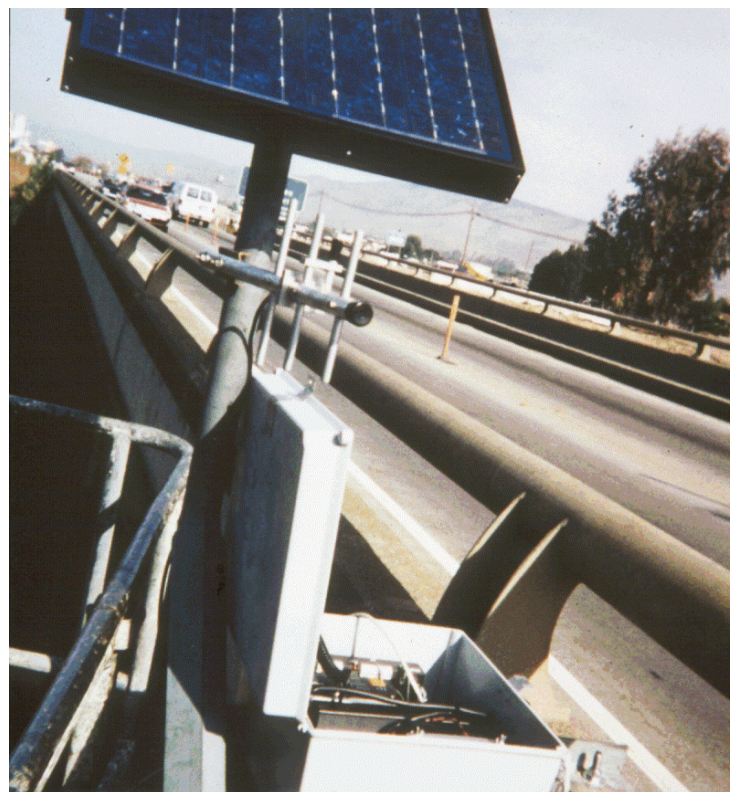
Figure 7.17. Typical instrument shelter with data logger, cell-phone telemetry, and a solar panel/gel-cell for power.
