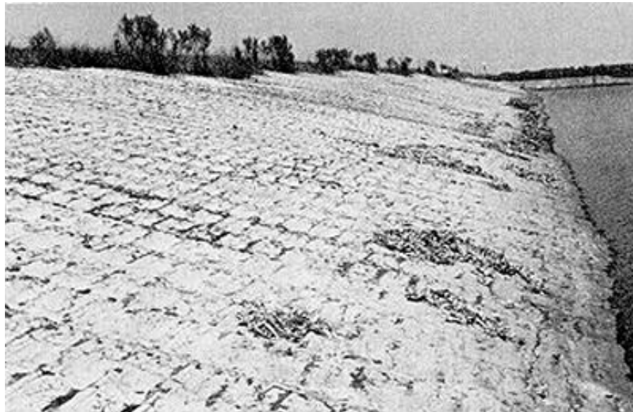
Figure 2.3. Soil cement placed in the plating method parallel to the slope (PCA).
