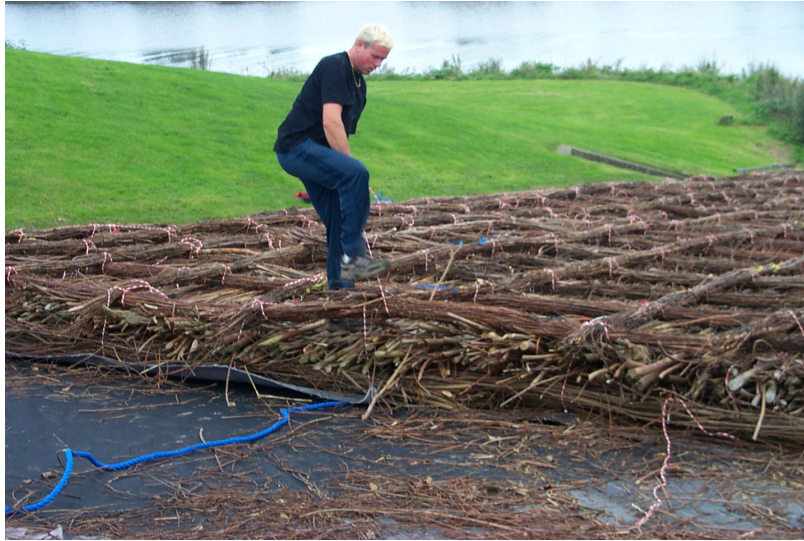
Figure 4.11. Fascine mattress: Fascine bundles tied on a base of woven geosynthetic fabric. (43)
