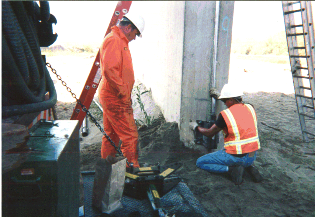
Figure 7.13. Installation of a sonar scour monitor on Salinas River bridge near Soledad, California (Highway 101) by CALTRANS.
