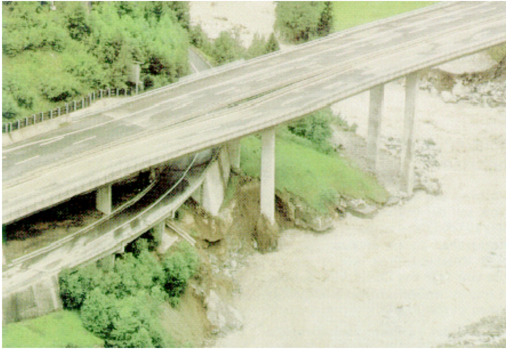
Figure 4.7. Reuss River bridge failure near Wassen, Uri Canton Switzerland, August 1987. (44)
