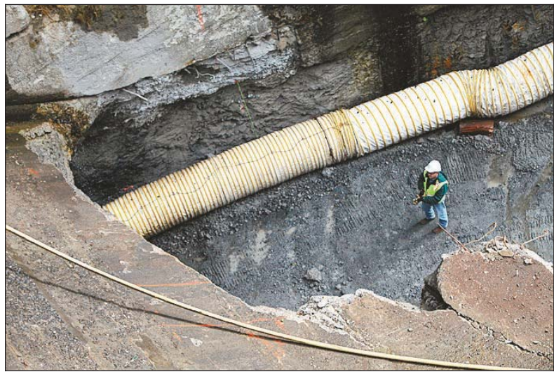
A construction worker prepares to enter a hole that will allow water to flow below the Condit Dam, emptying the reservoir behind it.
