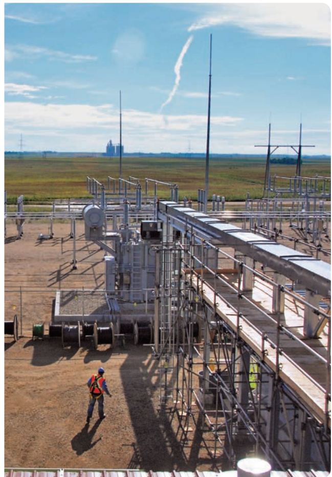
SaskPower is expected to invest $10 billion in the next 10 years to revitalize infrastructure and meet new load growth.
