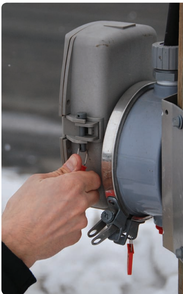
The replacement of existing meters with over 500,000 smart meters will help customers better track their power consumption.
