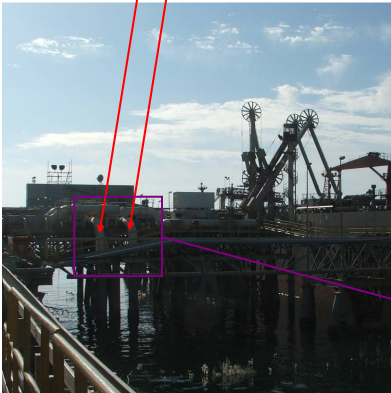
Site Photo 4. Two 48-inch incoming sea lines
