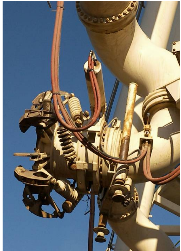
Site Photo 12. Loading arm connector for the tanker
