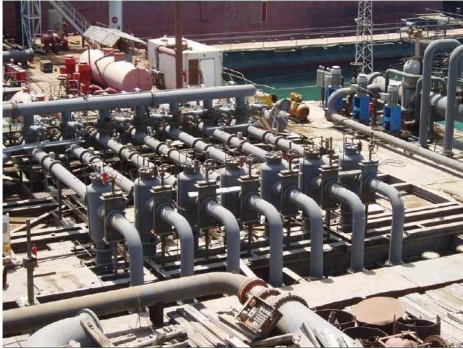
Site Photo 35. Condition of KAAOT platform prior to explosion
