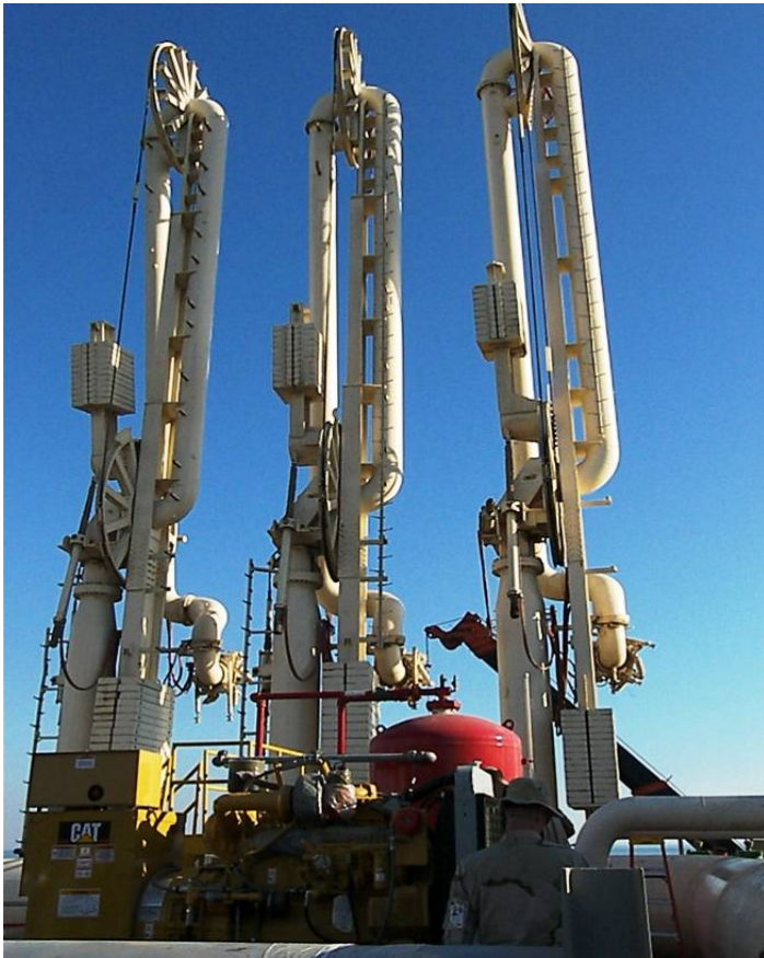
Site Photo 11. Loading arms in stand-by position
