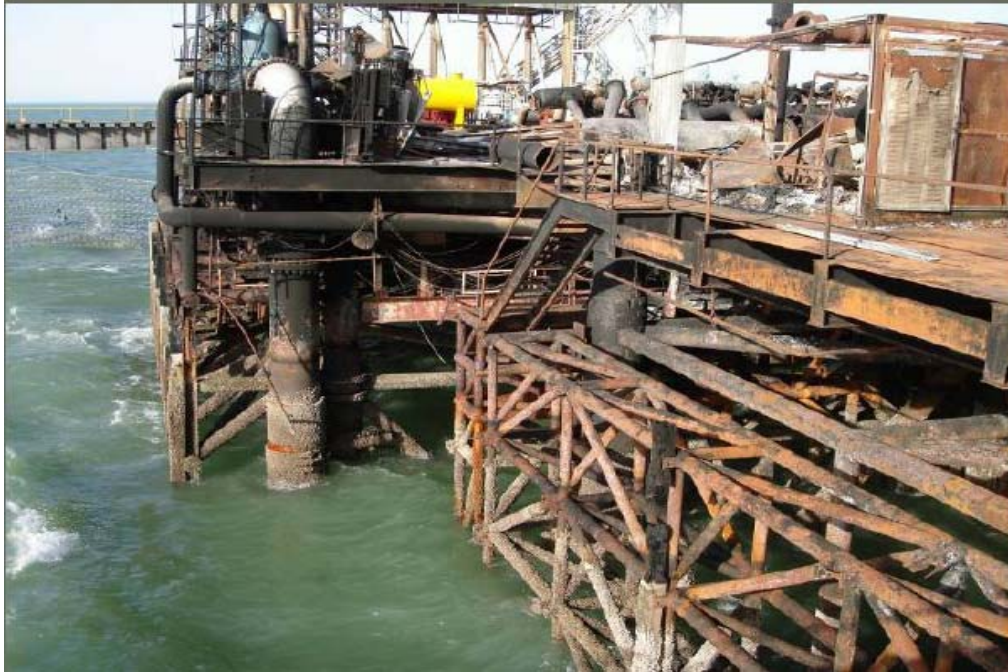
Site Photo 37. Condition of KAAOT platform after the explosion
