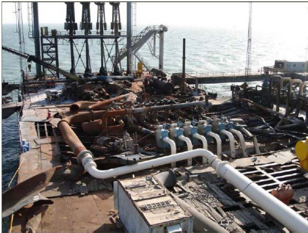
Site Photo 36. KAAOT platform after the explosion
