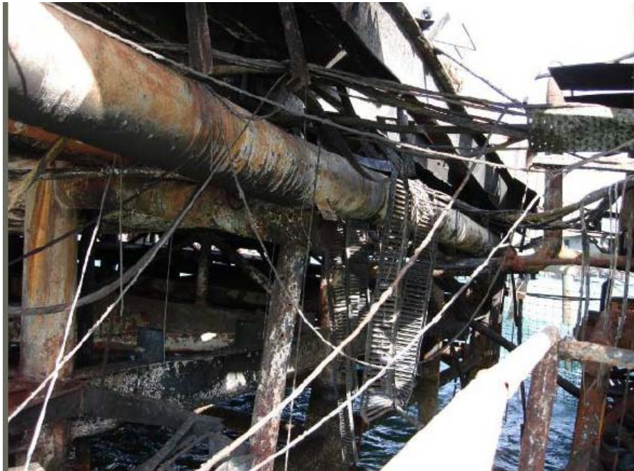
Site Photo 38. KAAOT platform after the explosion
