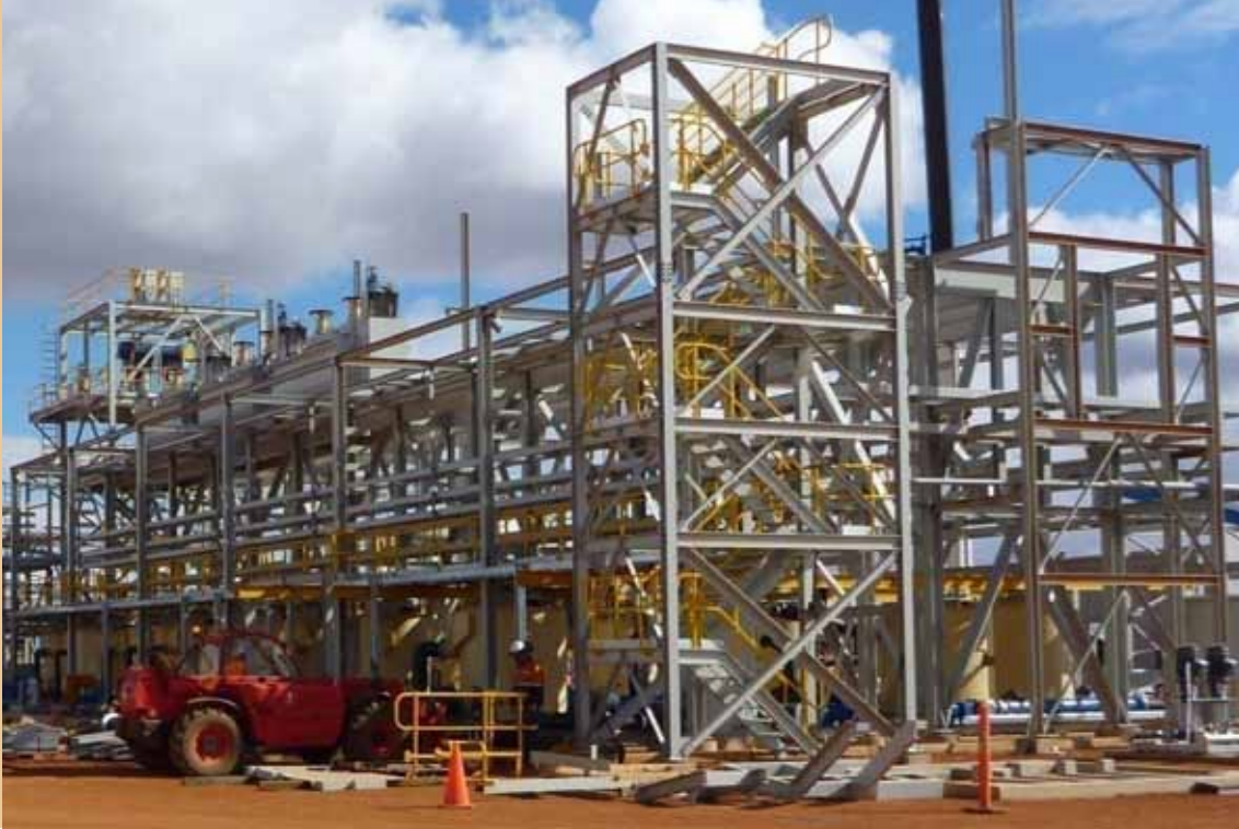
Construction of the concentration plant at Mount Weld rare earth project, Western Australia (Lynas Corporation Ltd)
