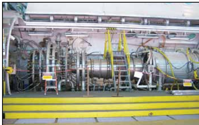
CAH with Freejet Nozzle Installed
