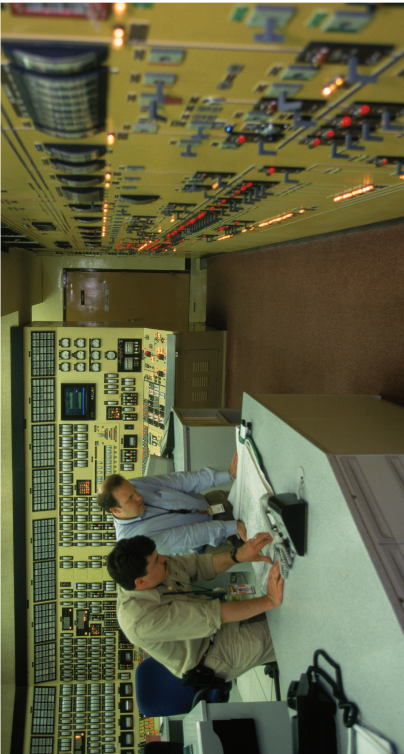
Nuclear power plant control room
