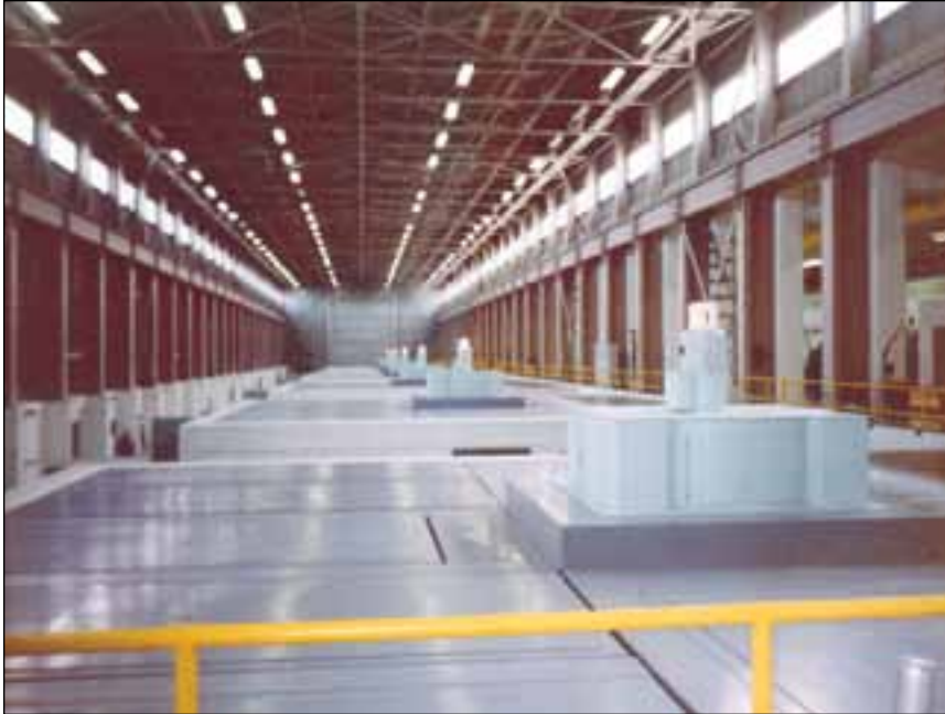
The interior of Kelsey Generating Station's powerhouse
