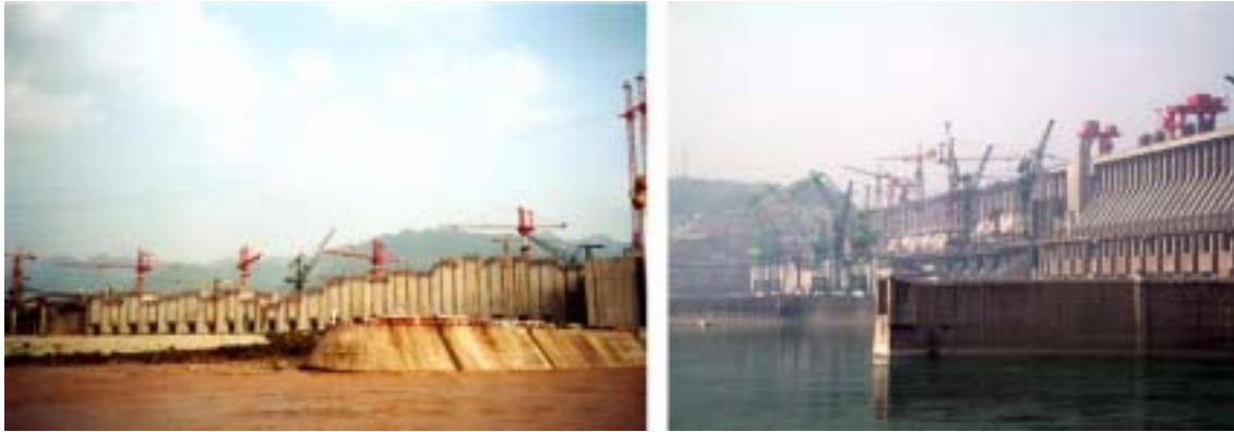
Figure 4: Images of the Three Gorges Dam construction. On the left, works on the left bank section of the dam, in September 2001 (Credit: Benjamin Lyons); on the right, works in the right bank dam, in April 2006 (Credit: Kay Young).
