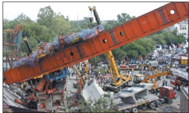
Figure 12.19: A section of an under-construction Delhi Metro flyover in the capital's Lakshminagar area collapsed and fell on a bus, killing at least two persons. (Source: blogs.reuters.com).
