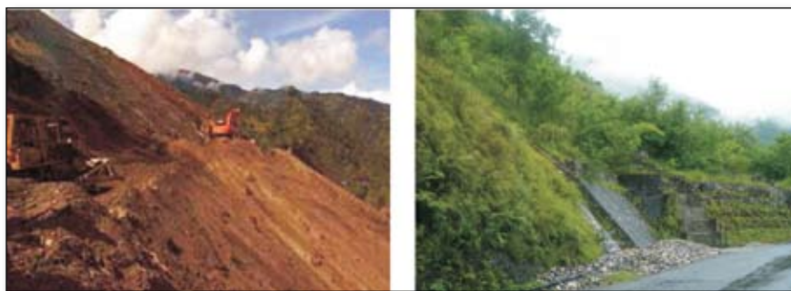
Figure 10.12: Failed slope at Krishnabhir in 2000 (left) and stabilized Krishnabhir in 2009 (right) 12
