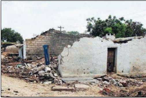
Figure 3.18: More than 1.22 lakh houses and over 13,000 huts were damaged, fully or partially, owing to the rain and floods in Raichur district, Karnataka (Source: The Hindu).
