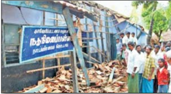
Figure 3.22: The collapsed Nattankottai Panchayat Union Primary School, near Krishnagiri (Source: The Hindu).
