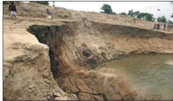
Figure 3.8: Collapse of part of flood control embankment at Raniganj point near Sirajganj town due to erosion by the Jamuna River (Source: The Daily Star).
