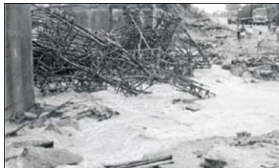
Figure 3.21: Collapsed scaffolding of the construction site of a bridge under construction across the Vahini River on the Hosur–Bagalur road in Bangalore (Source: The Hindu).
