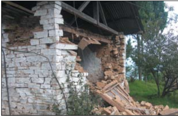
Figure 9.13: Damage to buildings the 21st September earthquake (Source: SQCA Bhutan).
