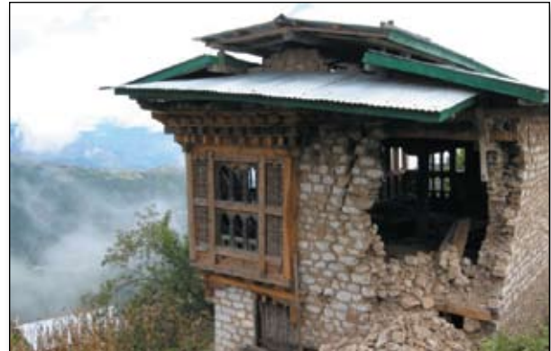
Figure 9.14: Damage to buildings during 21st September earthquake (Source: SQCA Bhutan).
