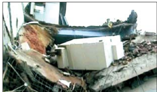
Figure 12.20: Collapsed part of City Center in Faridabad (Source: NDTV News).
