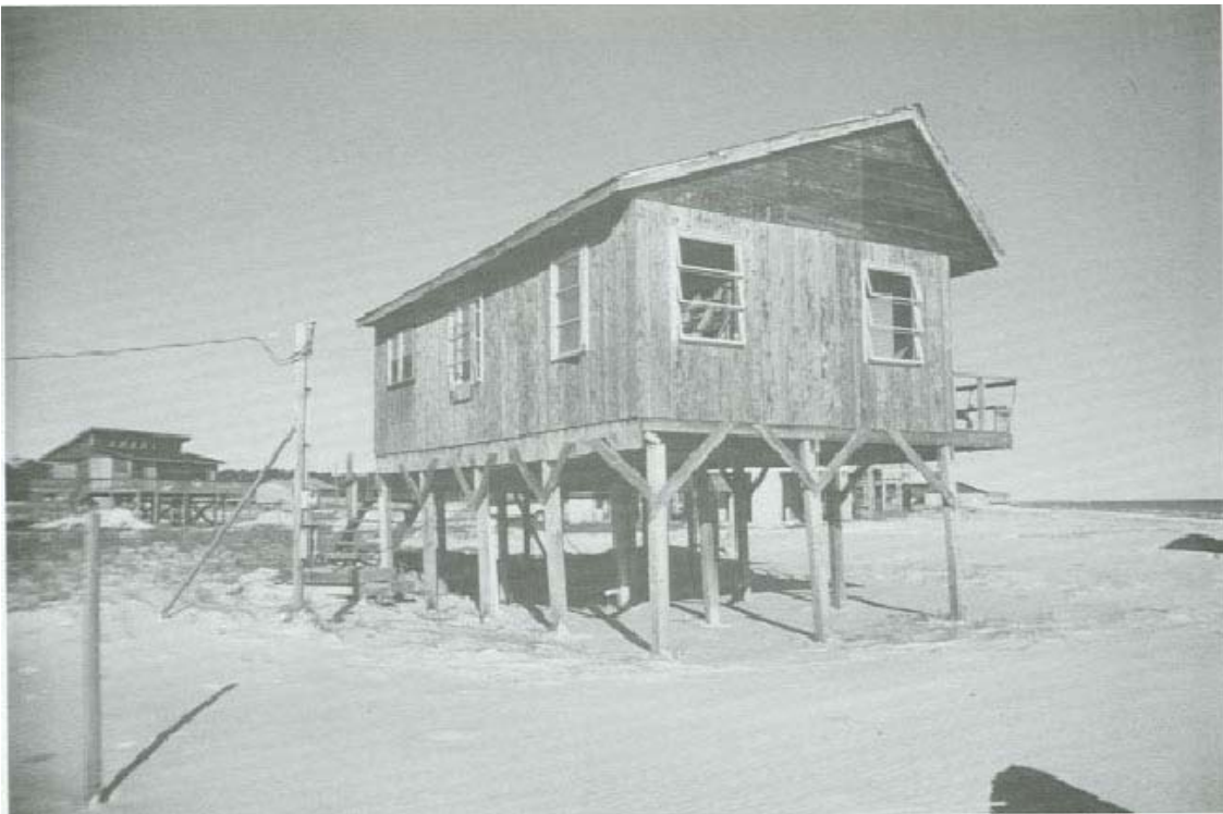
FIGURE 50. Pile-supported dwelling with inadequate pile to beam connections and insufficient pile penetration leans following wind loads and scour.
