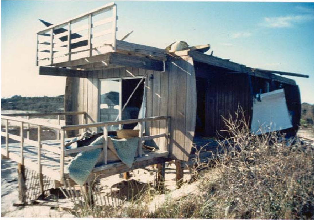
FIGURE 47. Barrel-shaped house destroyed by wind.
