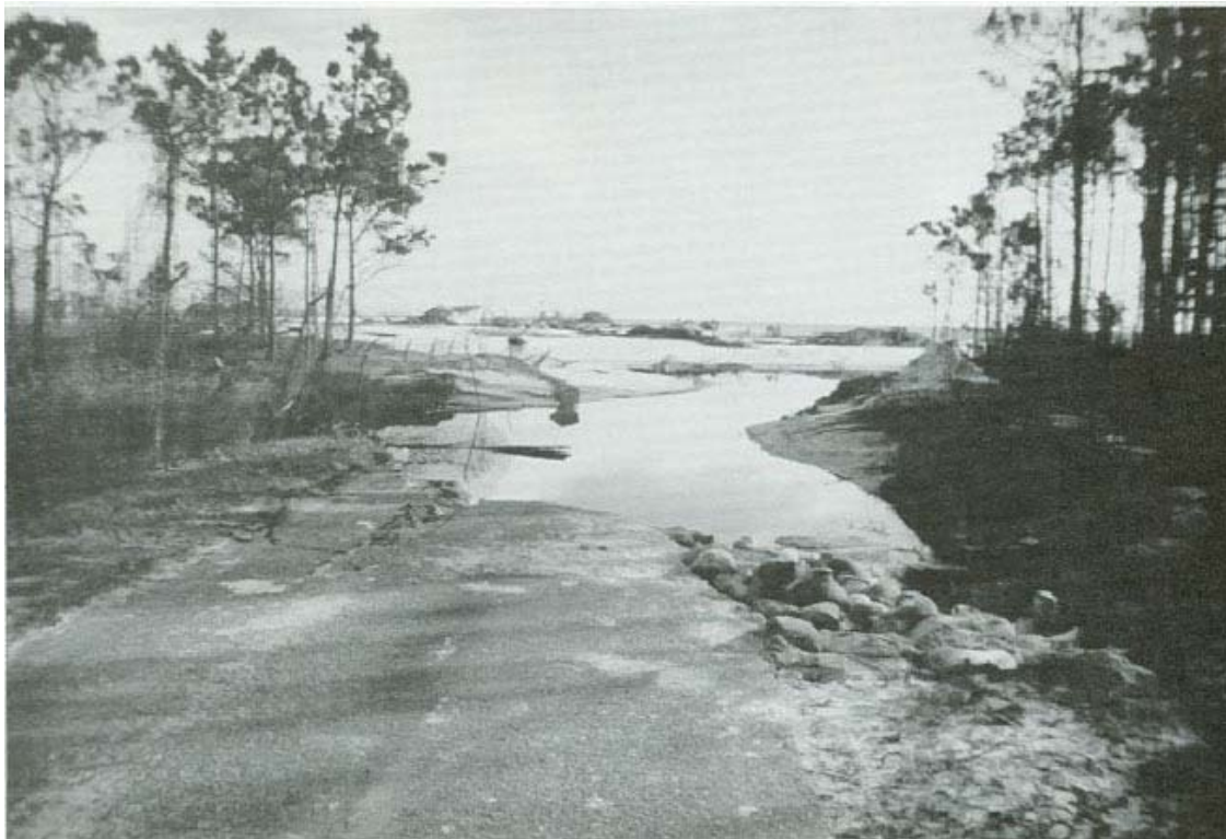
FIGURE 20. Cape San Blas beach access road destroyed.
