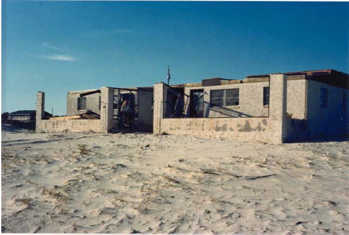
FIGURE 51. Duplex sustained major structural roof damage.
