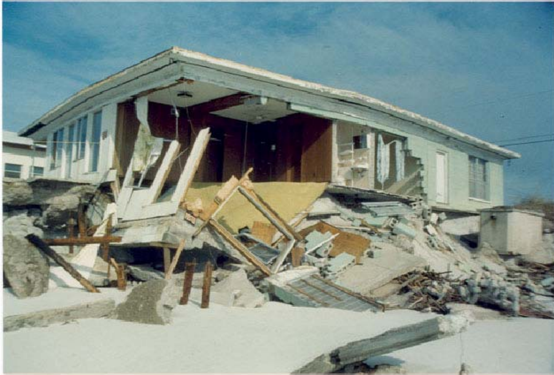
FIGURE 9. Slab-on-grade dwelling partly destroyed, Panama City Beach.
