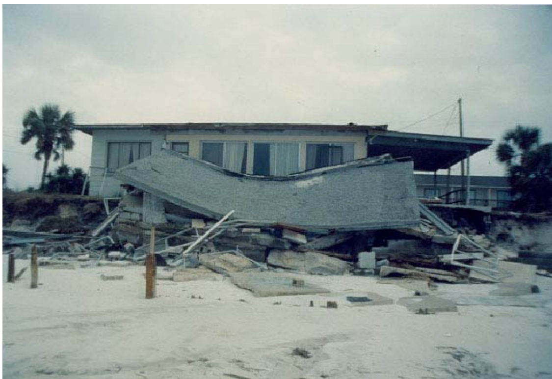
FIGURE 12. Seaward room destroyed on Mexico Beach dwelling.
