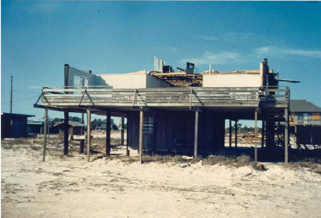
FIGURE 46. St. George Island beach Dwelling destroyed by wind.
