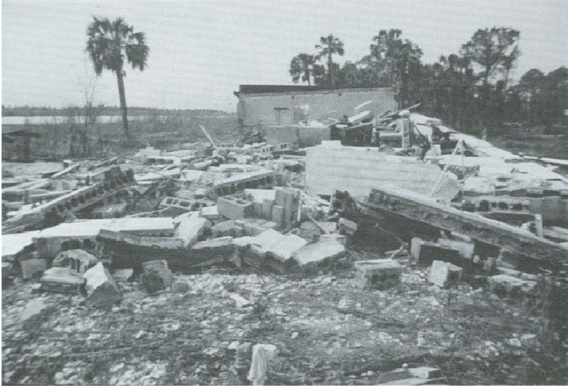
FIGURE 30. Concrete block commercial building destroyed by waves.
