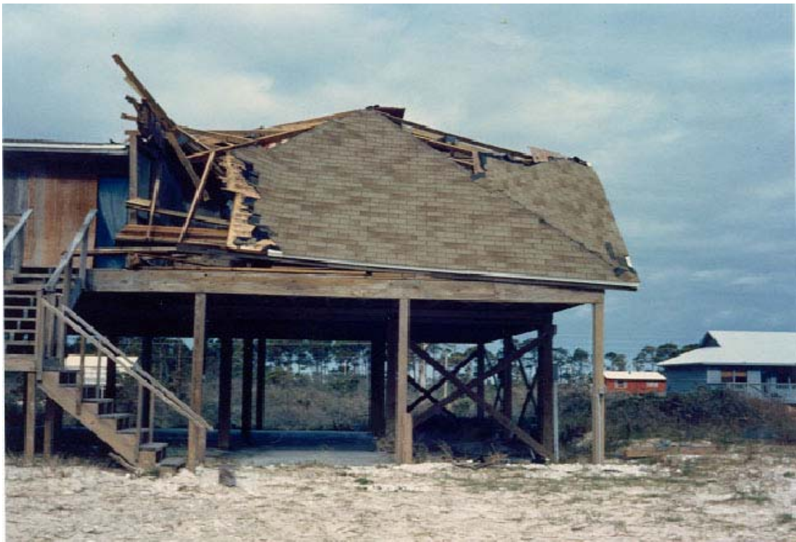
FIGURE 44. Gorrie Drive dwelling's roof collapsed.
