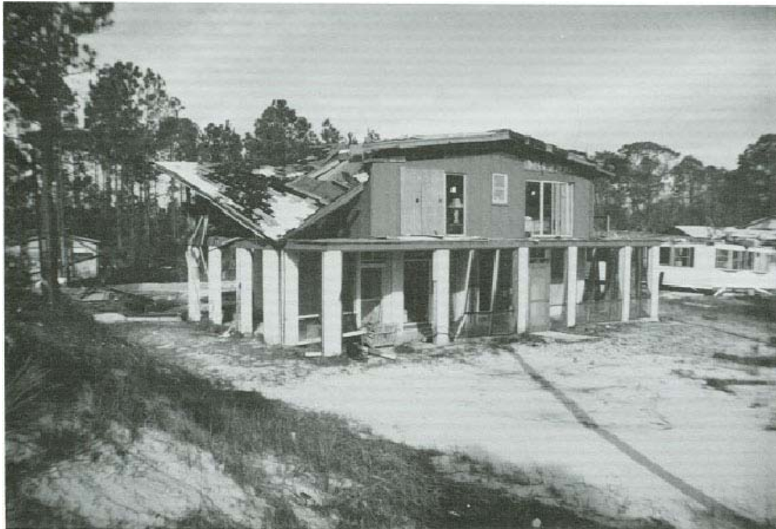
FIGURE 23. Dwelling damaged by wind and flooding.
