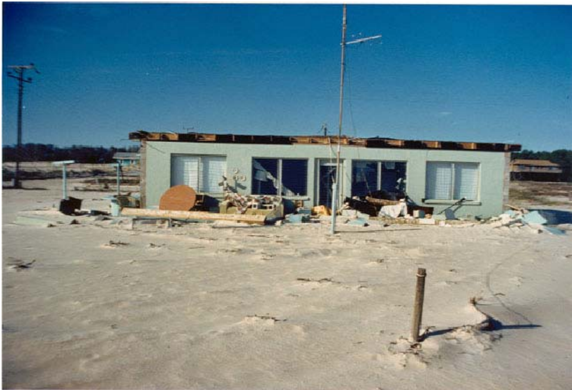
FIGURE 48. Structural roof damage due to wind and concrete block porch destroyed by waves.
