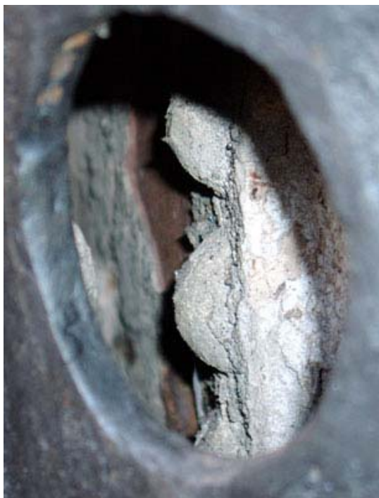
A crust of scale exists on the water side surfaces of this boiler. If that was not bad enough, as is to be expected, under the scale is some less than healthy corrosion.
