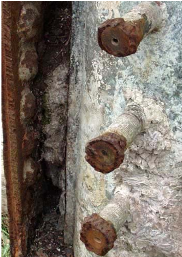
A frightening photo - this boiler was in daily use in this condition. The scale is so bad the water space from the foundation ring up is blocked solid. Not surprisingly the inner firebox shows signs of rippling - this boiler has, thankfully, been condemned! But it need not have ever been in this condition.....
