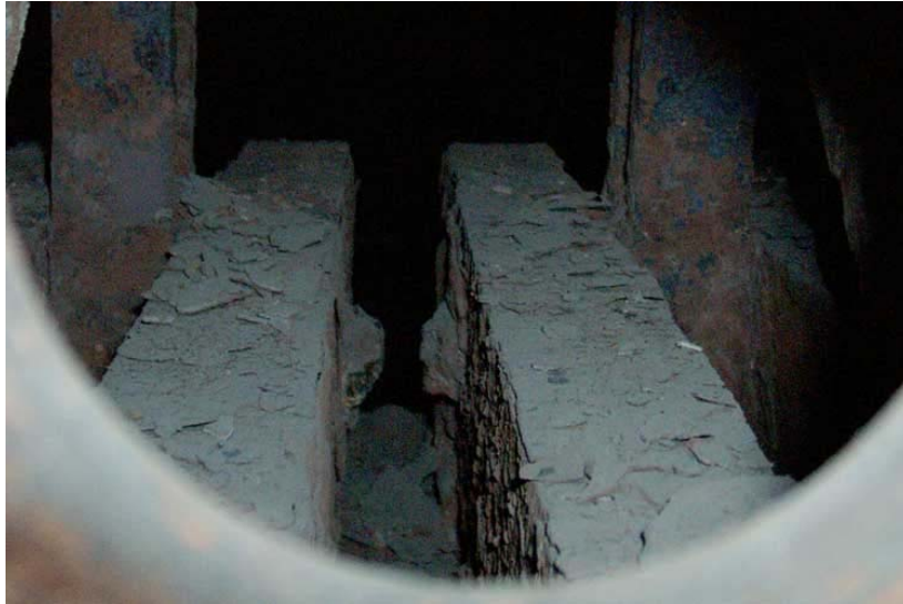
Corroded and scaled girder stays in a boiler which has seen better days!
