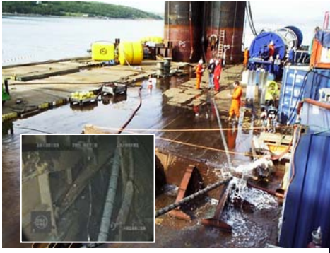
The cable cutting rig trials on Giant 4 suction anchors (top) acting against an opposite set actual underwater cutting (inset)
