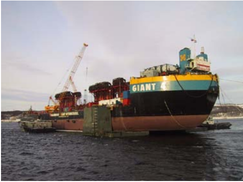
Giant 4 with the Kursk slung underneath awaits entry into the floating dock at Rosljakovo – two specially designed sinkable pontoons were deployed to raise Giant 4 for the necessary clearance into the floating dock
