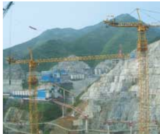
The two cranes on site are shortly to be joined by a third unit.
