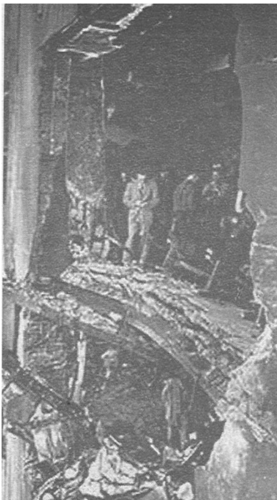
One of the R-25 engines, and part of the landing gear, went through the building, tearing a hole 18 by 20 feet
