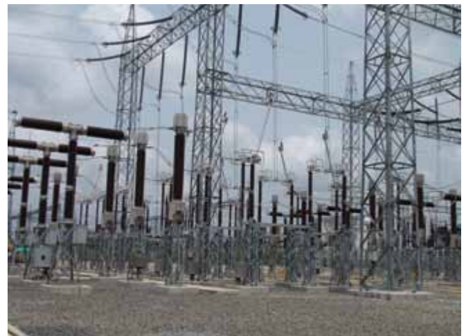
Switchyard – Afam Power Plant
