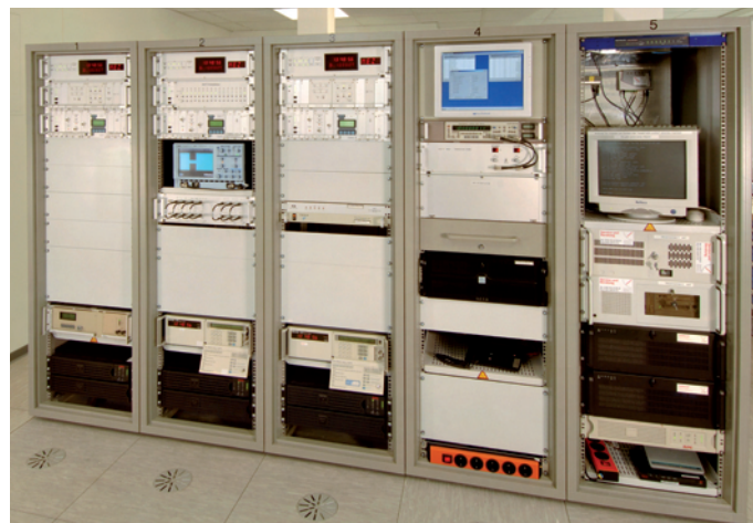
Figure 8: DCF77 control facilities of PTB. The atomic clocks, the drive signal generators and the electronic converters are installed in the racks 1 to 3. Rack 4 contains the local measuring equipment and the interface for communication between Mainflingen and Braunschweig. Rack 5 contains the interface for feeding in alarm and weather information.
