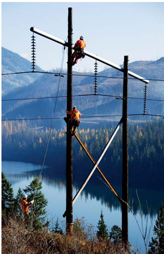
The $110 million Okanagan Transmission Reinforcement Project is the largest capital project ever undertaken by FortisBC.
