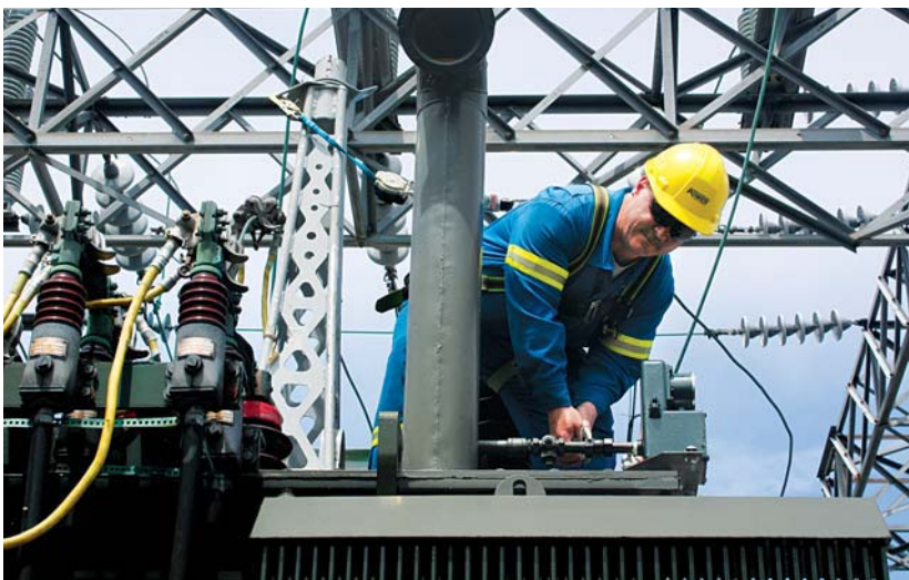
Almost $74 million, before customer contributions, was invested in capital projects in 2009 to upgrade and modernize the utility's electricity system.
