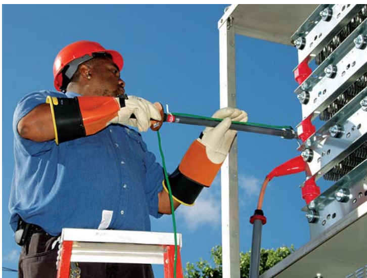
Caribbean Utilities is one of the most reliable and efficient utilities in the Caribbean region.
