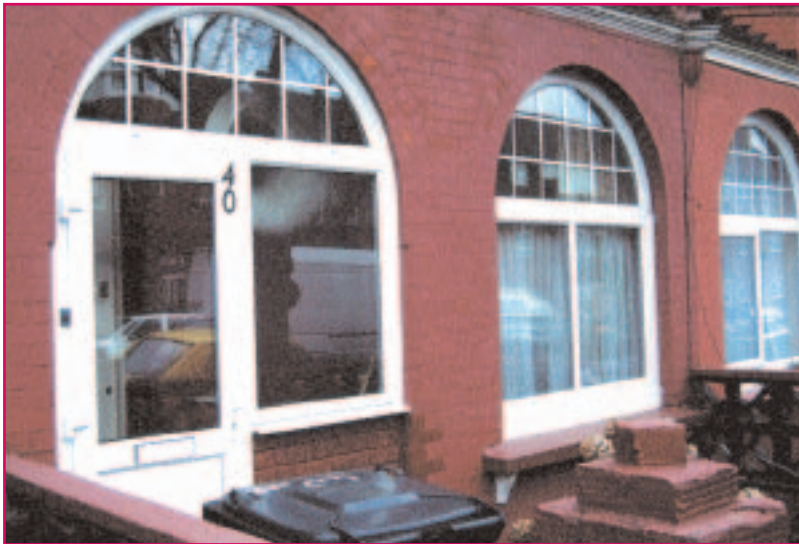
PVCu porch enclosure and inauthentic PVCu windows.
