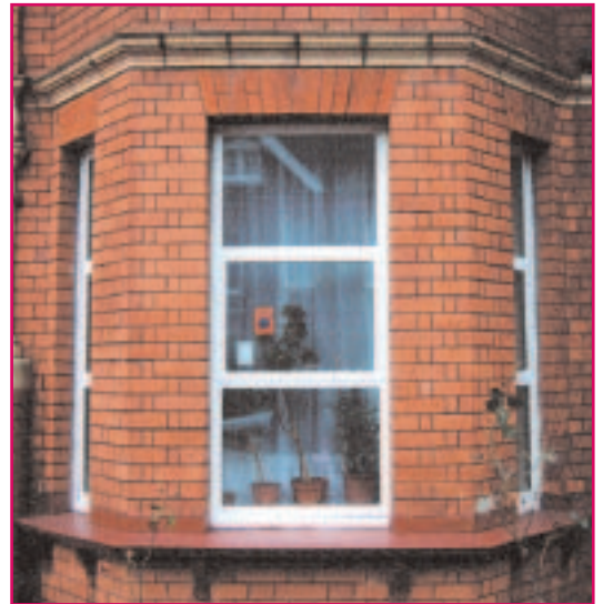
PVCu windows - with poor horizontal proportions.
