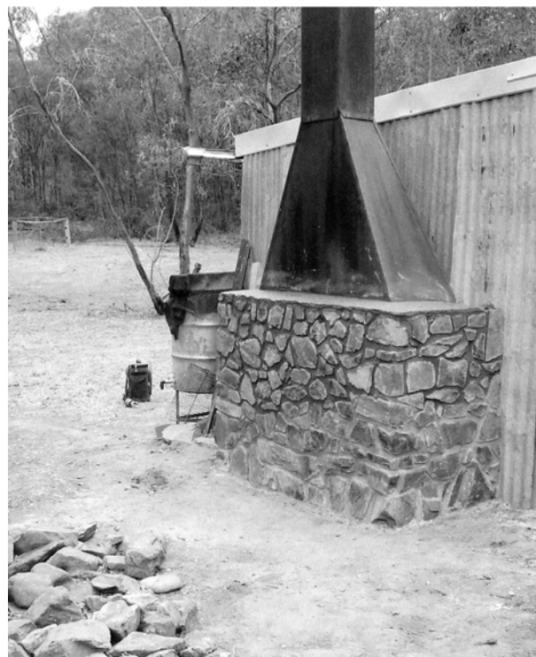
Laverty's hut chimney, after works. A good example of why Brad and his team are in demand with other HMOs wanting rockwork done. Photo courtesy of Brad Cooksey
