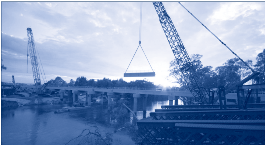
The new rail bridge was constructed in prefabricated sections over a four-day period in January 2007 (Photo DOTARS)
