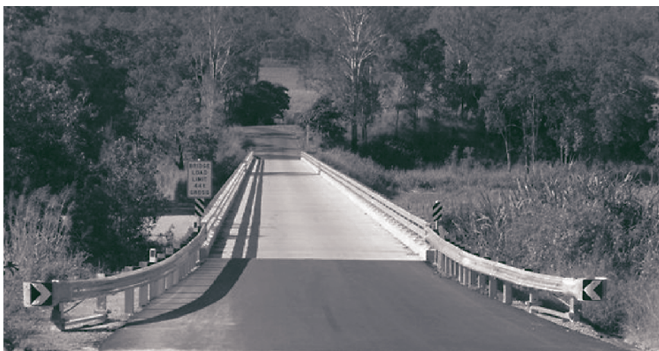
The $2.3m recently upgraded Higham's Bridge on Owens Creek Loop Road off the Mackay Eungella Road, Queensland (Photo DITRDG)
